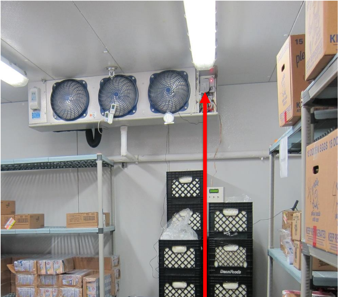
In Walk in Cooler
