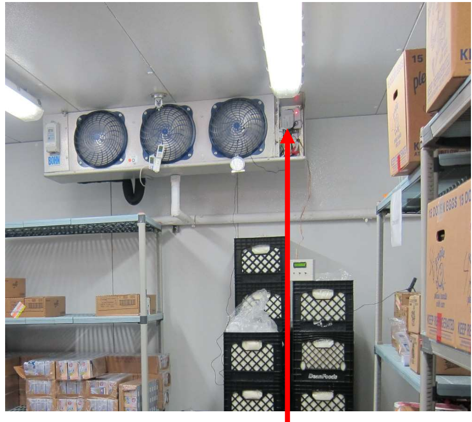
In Walk in Cooler
